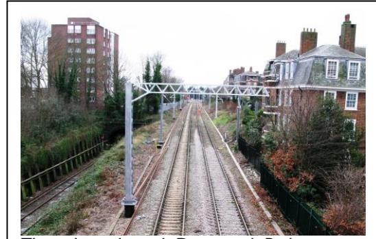
The railway through Dartmouth Park awaits the overhead wires on 2 nd February 2017.
