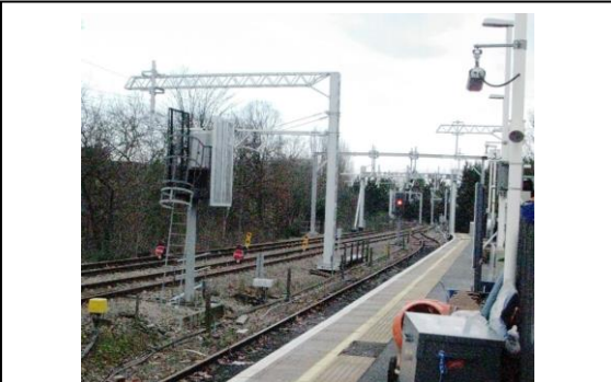
Gospel Oak on 13 th January 2017. The platform line has yet to receive overhead wires.
